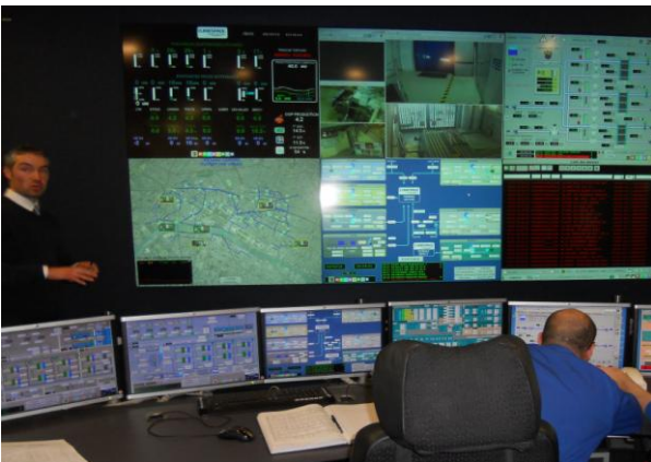
Climespace control centre - monitors all the buildings It services from a central point
